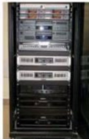
TASCAM, Sennheiser and QSC equipment in the rack
